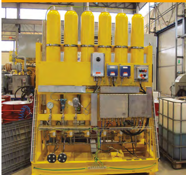
Hydraulic station with ATEX components.
